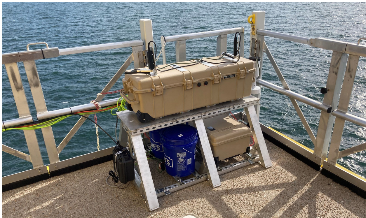
Figure 2. The core ATOM system components installed on the CVOW turbine platform.
